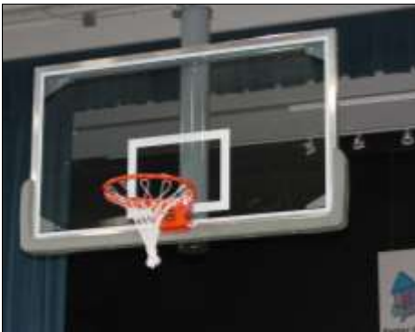
March Madness came early with installation of retractable basketball backstops, courtesy of the Kivwanis Cares for Kids Auction.
